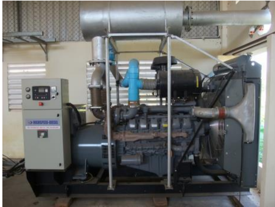
Dual fuel gas-diesel engine at Golden Daun Keo rice mill, Battambang, Cambodia, 2014-12-20
