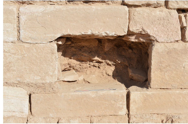
Fig. 25. Sounding H deep. Location of the fill (35332) after removal. The cavity left behind did not reveal anything other than the interior of an ordinary wall. Looking north-west.
