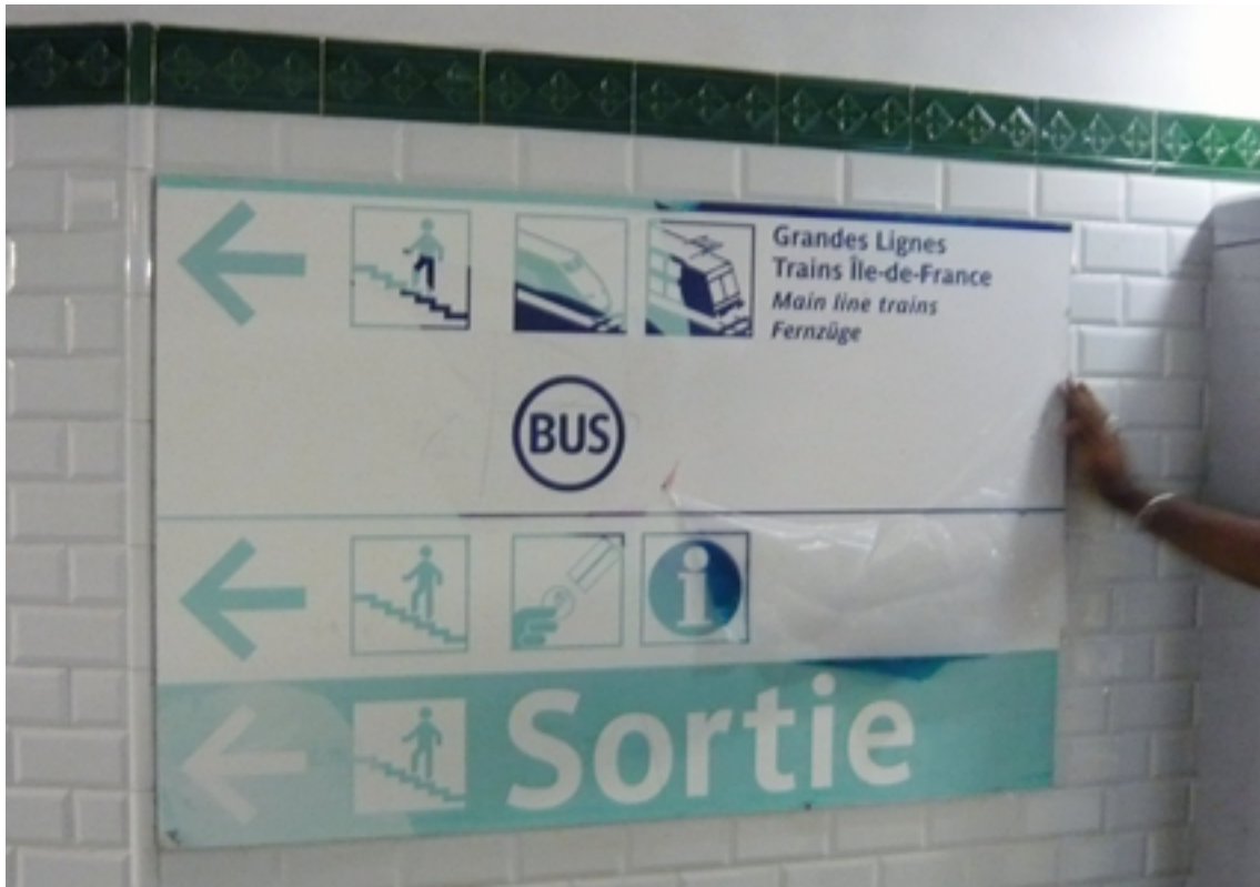
Figure 2. A discolored signboard
