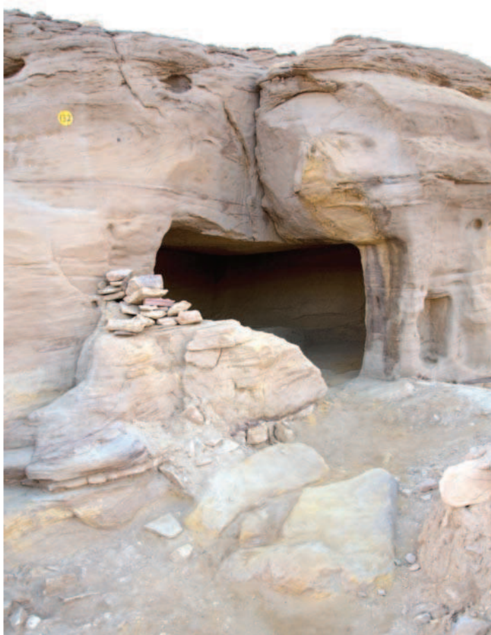
Fig. 7 View of the rock-cut chamber IGN 132a showing the collapse of the ceiling
