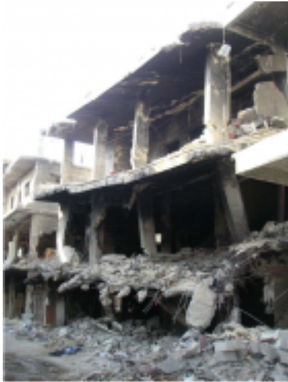
A damaged building, new camp, Nahr el-Bared, November 2007.
