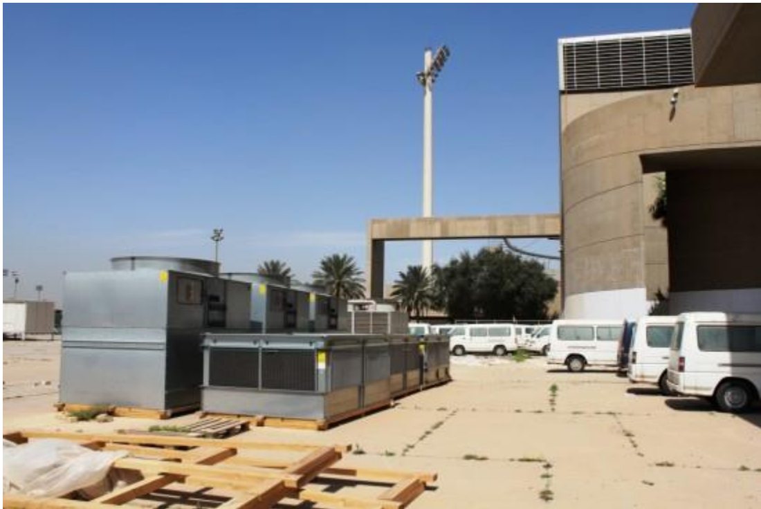
Fondation Le Corbusier/ ADAGP/ Caecilia Pieri, 2012. Modifications due to the ongoing renovation: air vents for AC in front of the façade.
