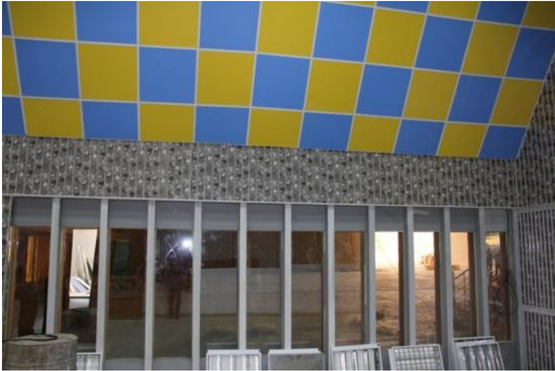
Fondation Le Corbusier/ ADAGP/ Caecilia Pieri 2012. Modifications due to the ongoing renovation: internal hanging ceilings.
