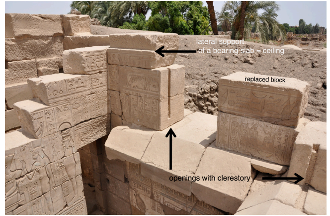
Constructional details of the Ptolemaic clerestory lighting and roofing of the courtyard. One of the scattered blocks has been replaced on the top of the wall. © CNRS-CFEETK/Pierre Zignani
