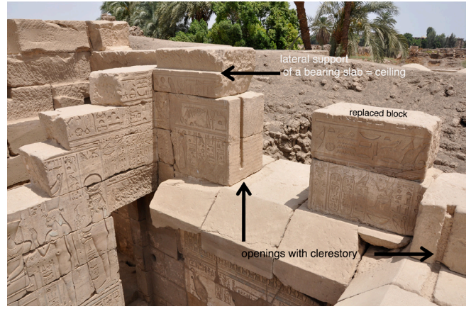
Constructional details of the Ptolemaic clerestory lighting and roofing of the courtyard. One of the scattered blocks has been replaced on the top of the wall. © CNRS-CFEETK/Pierre Zignani
