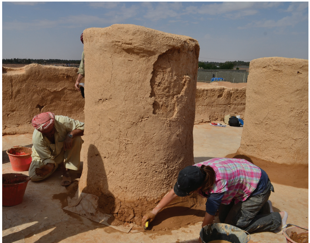
Figure 18: Building 1 - Earthen coat protection applied above geotextile at the base of a column (J. Schiettecatte - Saudi-French archaeological mission in al-Kharj).
