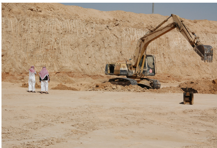
Figure 137: Al-Hayāthim ‘palaeolake’. Excavator digging another 4.5 m-deep trench (Saudi French archaeological Mission in al-Kharj).
