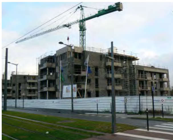
Illustration 33: Tramway of Valenciennes - Construction of a residential building on the outskirts of Denain - source : photo CETE Nord Picardie 2011
