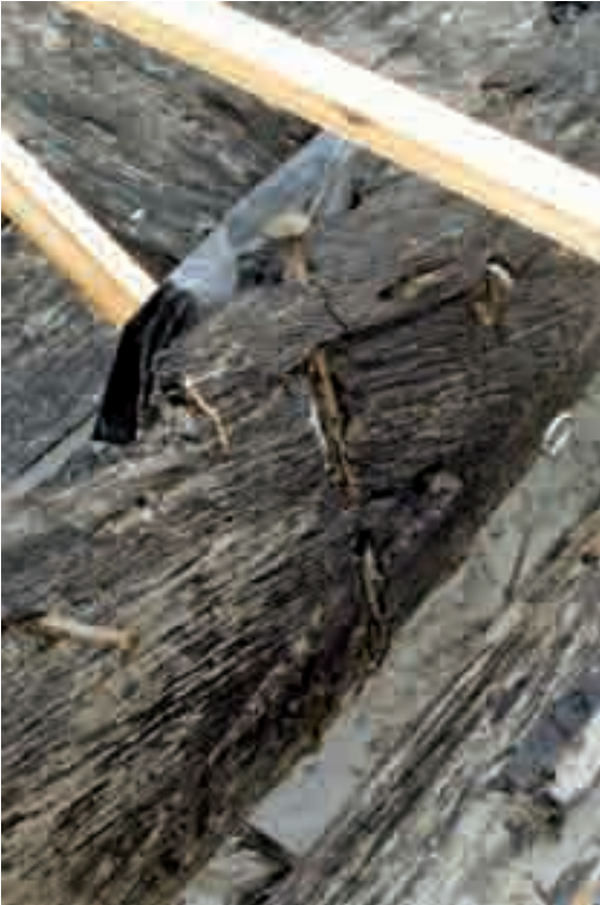
Fig. 2. Long nail running through scarf between two elements of the L-shaped chine (photo T. Penders, RCE).
