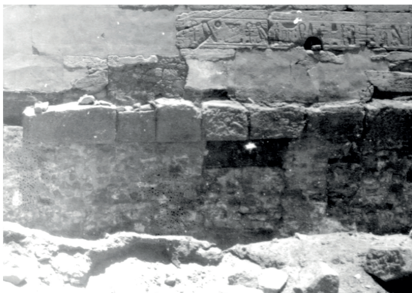
Fig. 9. Close-up of the unfilled gap of the point C of Fig. 1 in the foundations of the eastern wall of the Cachette Court. © CNRS-CFEETK 94495.
