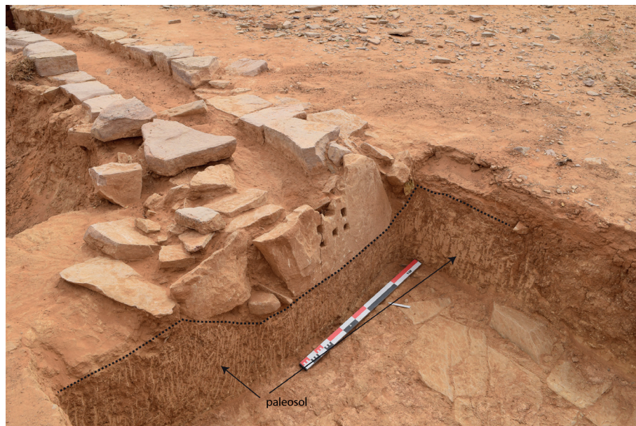
Fig. 7. The slab and the filter at the west end of channel L3014, ©MADAJ, R. Mensan.
