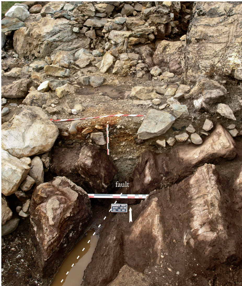
Fig. 9: Section indicating the fault in the dolomite bedrock at the junction of the spillway and the tail-race (photograph by N. Minvielle Larousse).
