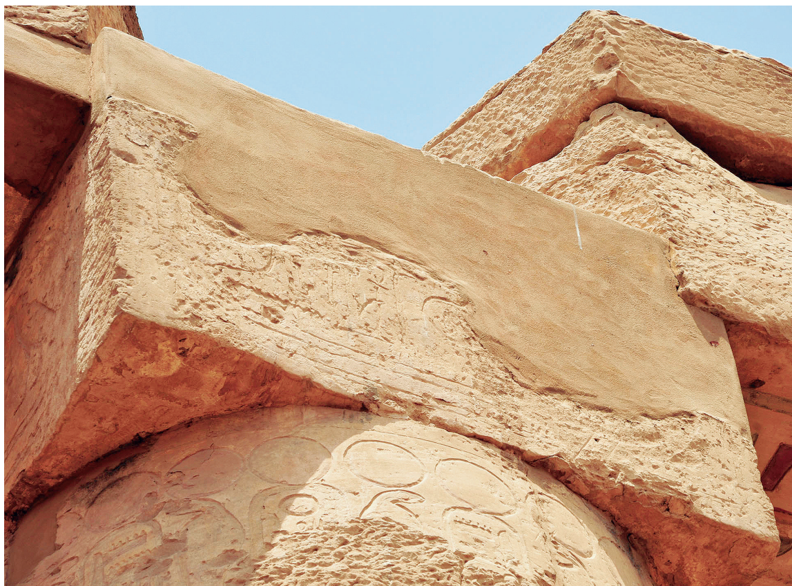
Fig. 1. Abacus 59 south covered in large part with cement.
