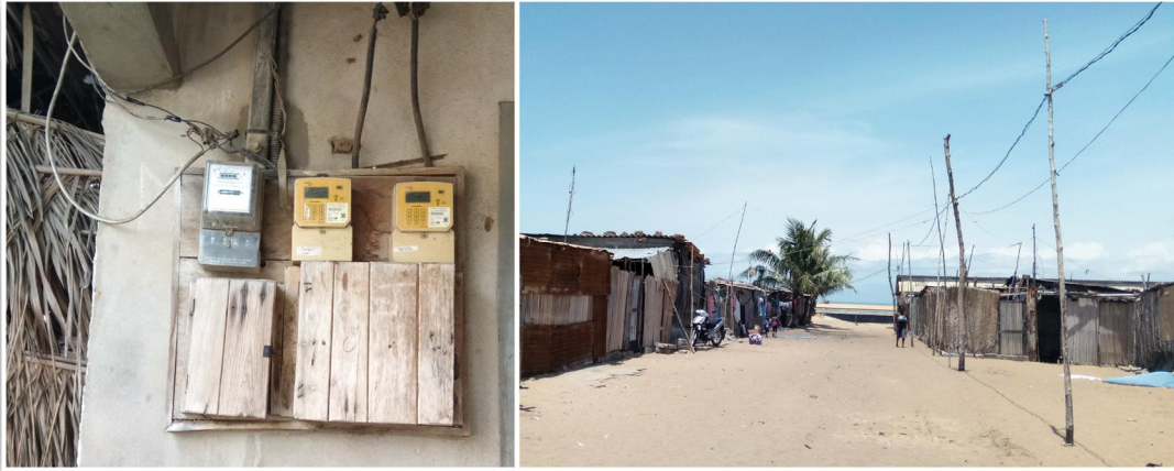
Figure 5: Metres installed in the neighbour's house and DIY connection.
