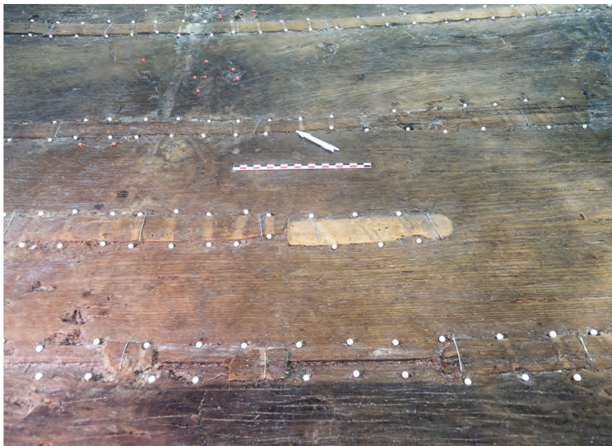
II.22 Pogled na popravak pukotine u sredini kobiličnog elementa P2 View of the crack repairs in the middle of keel-like timber P2 (fotografija / photo by: Ph. Groscaux)
