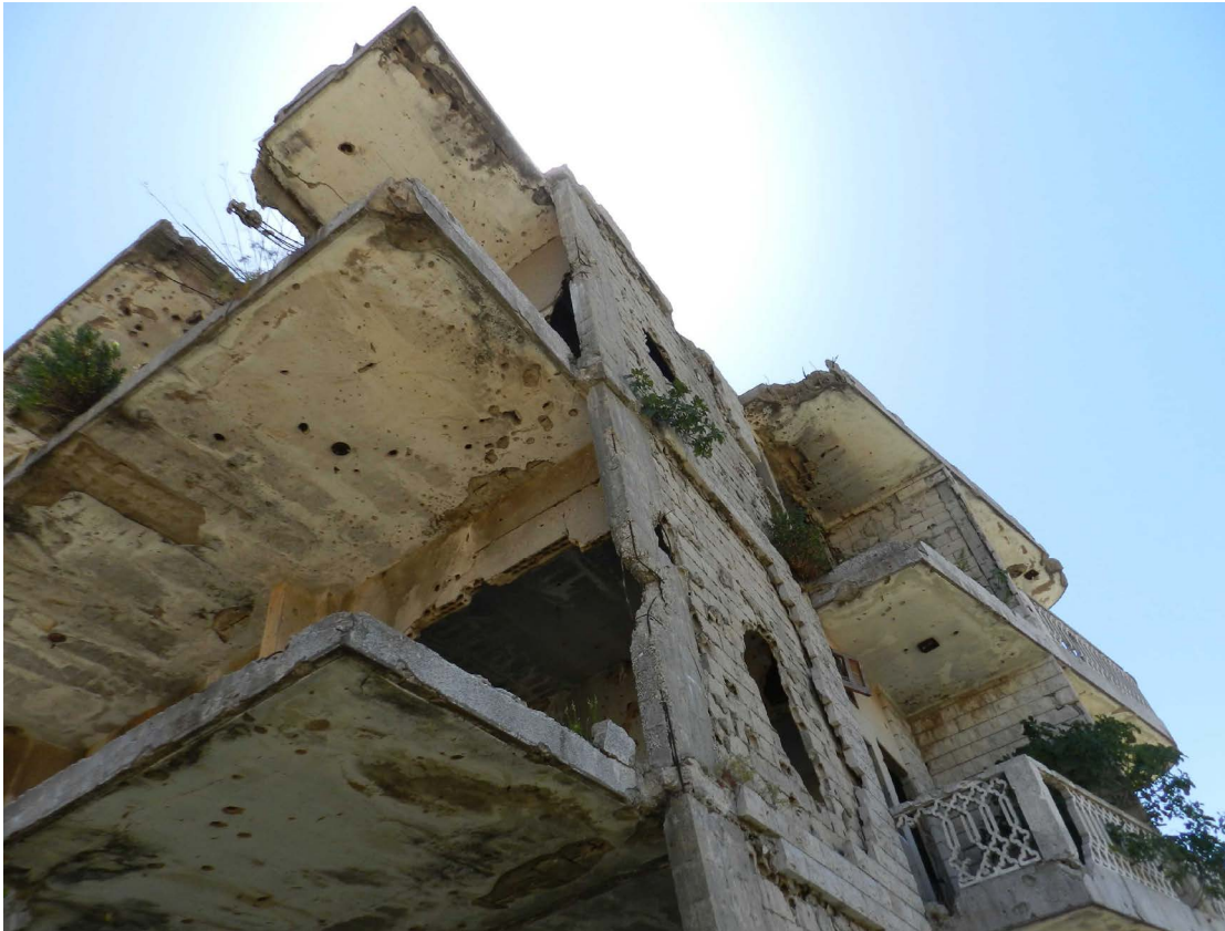
Figure 4. Qleiaat: building destroyed during inter-Christian clashes at the end of the Lebanese civil war
