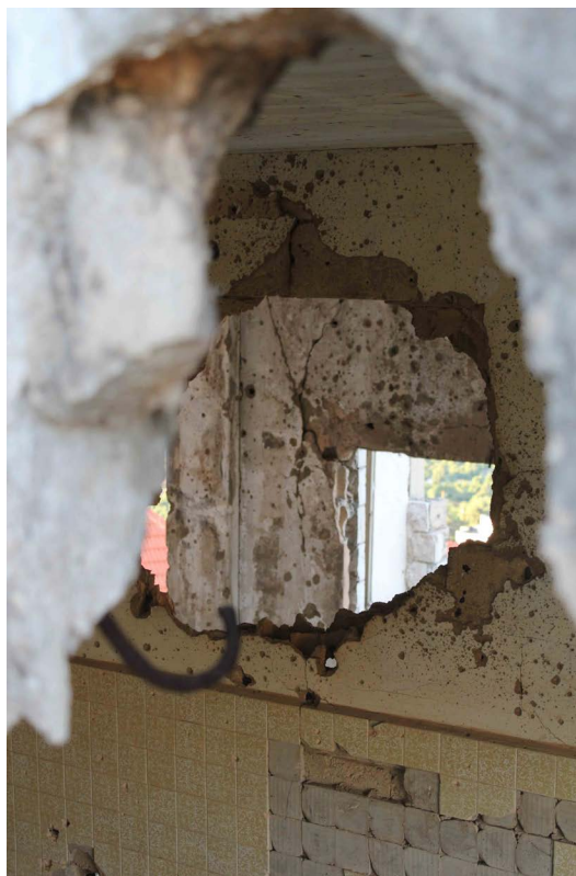
Figure 6. Qleiaat, upper portion of the village: holes in the walls from impacts of mortar shells
