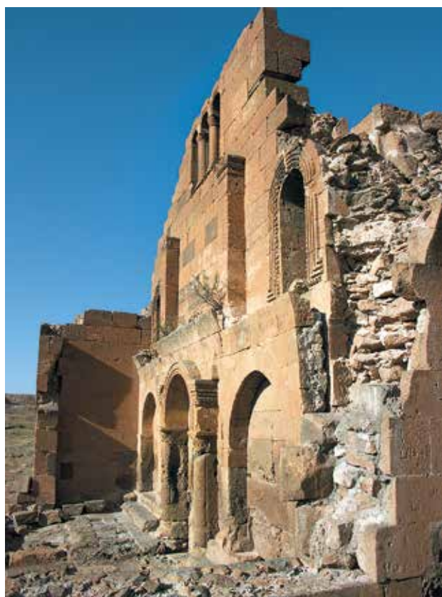
Fig. 5. Yereruyk basilica. Masonry leaning against the western facade for the addition of a new gallery, lowered (Photo: Author, LA3M, 2013).
