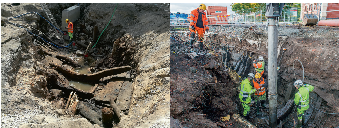
Fig. 2: In the left-hand picture we can see the stern with the first rider. The big concrete block is like an anchor that will hold the front of the new quay. In the picture to the right, the starboard side is visible. The big pipe is the suction digger that we used. (left-hand photograph, Annelie Karlsson, Swedish National Maritime and Transport Museums; right-hand photograph, Johan Runer).
