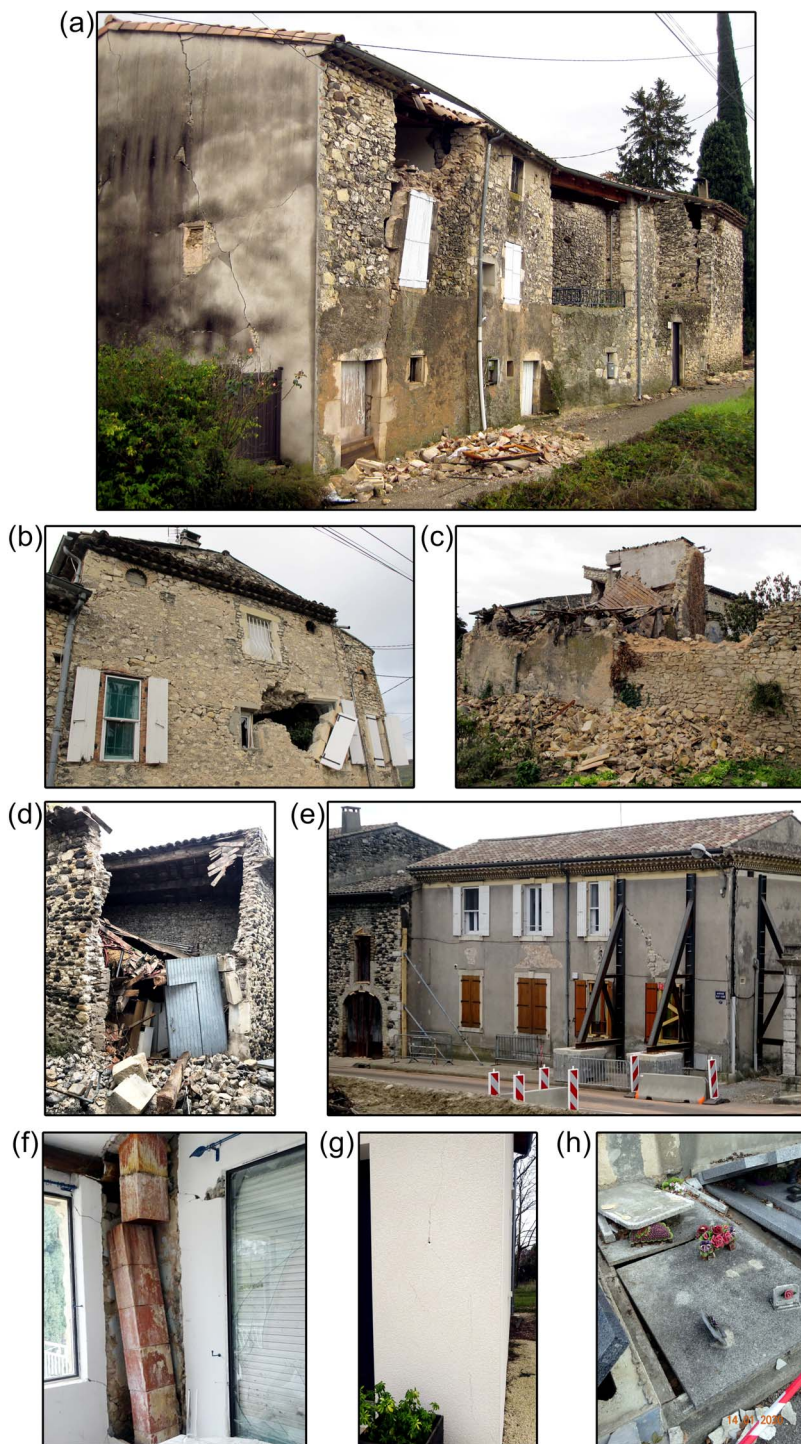
Figure 8. Types of damage observed in the zone of maximum intensity VIII, locality of Le Teil, from La Rouvière district (photographs a, b, c) to the Mélas district (photographs d and e), and on the road connecting the two districts (photographs f, g, h).
