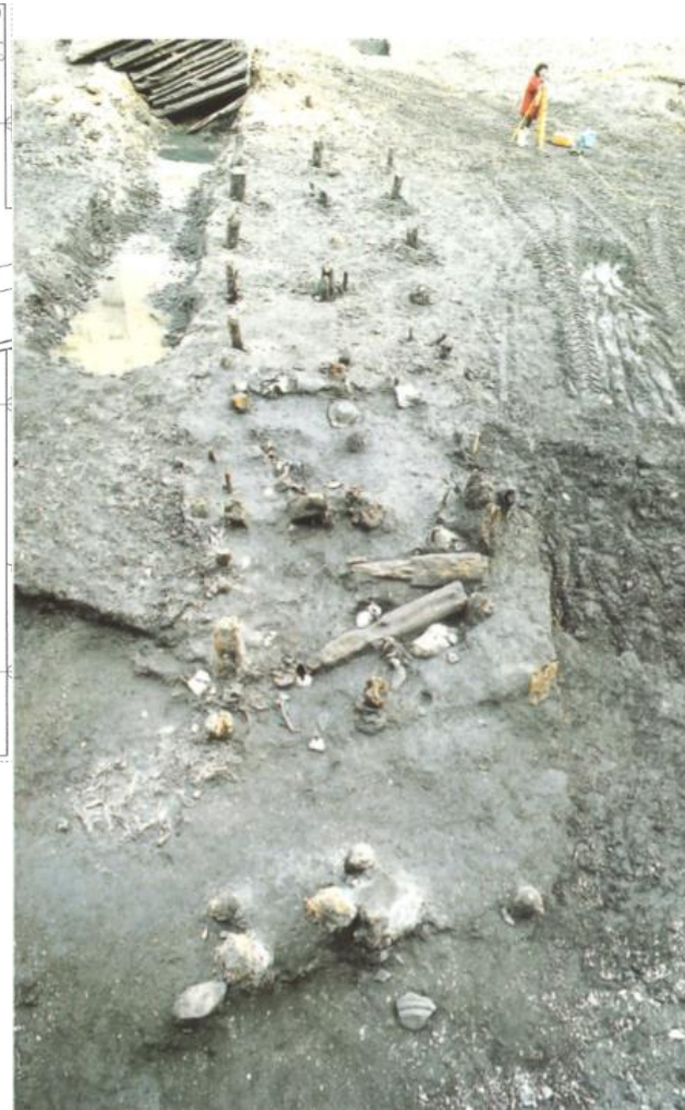
Support piles of the wooden landing stage. Jules-Verne excavations (M. Derain /AFAN)
