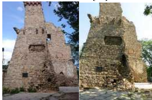
Fig. 9. Constantine tower in year 2015 (photo by K. Veprytska). Constantine tower in September 2016 [33]
