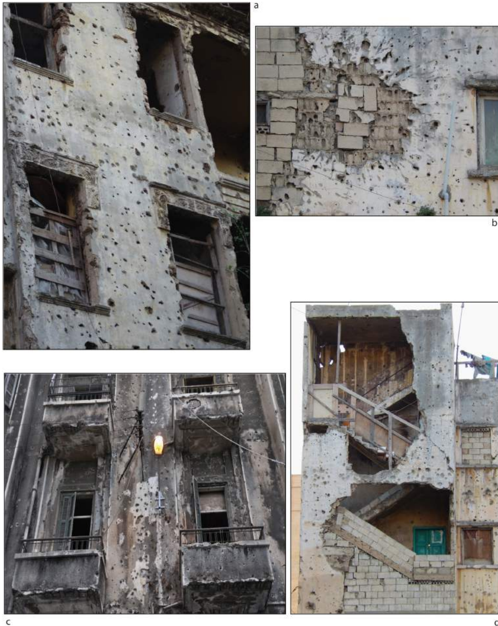
Figure 2: a, b, c: Beirut. Impacts of bullets on plastered façades. d: Beirut. Broken staircases and windows sealed with concrete blocks to protect the snipers.
