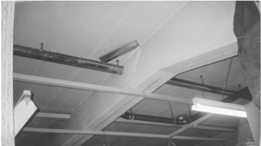
Figure 5.6 The installation of internal gutters, Ethnologisches Museum, Staatliche Museen zu Berlin, photographer: Hans-Joachim Radosuboff
