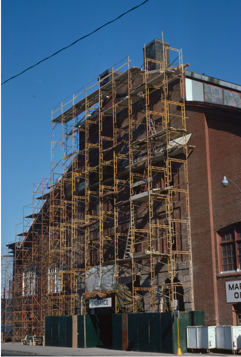
Figure 6.11. View of scaffolding on St. Lawrence Market. May 13, 1975. Courtesy of the City of Toronto Archives, Fonds 1526, File 16, Item 8.
