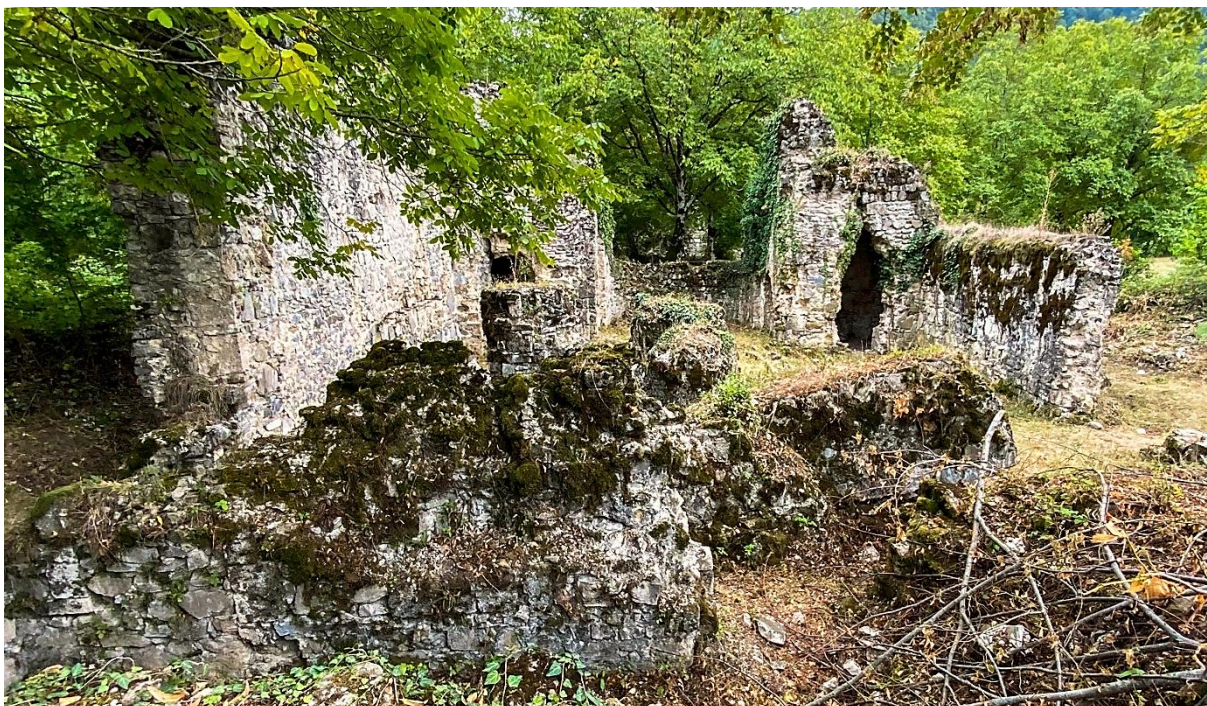
Fig. 5 (p. 396). Yeddi Kilsə. Western church, general internal view from west to east. Online photo Sefer Azeri.
