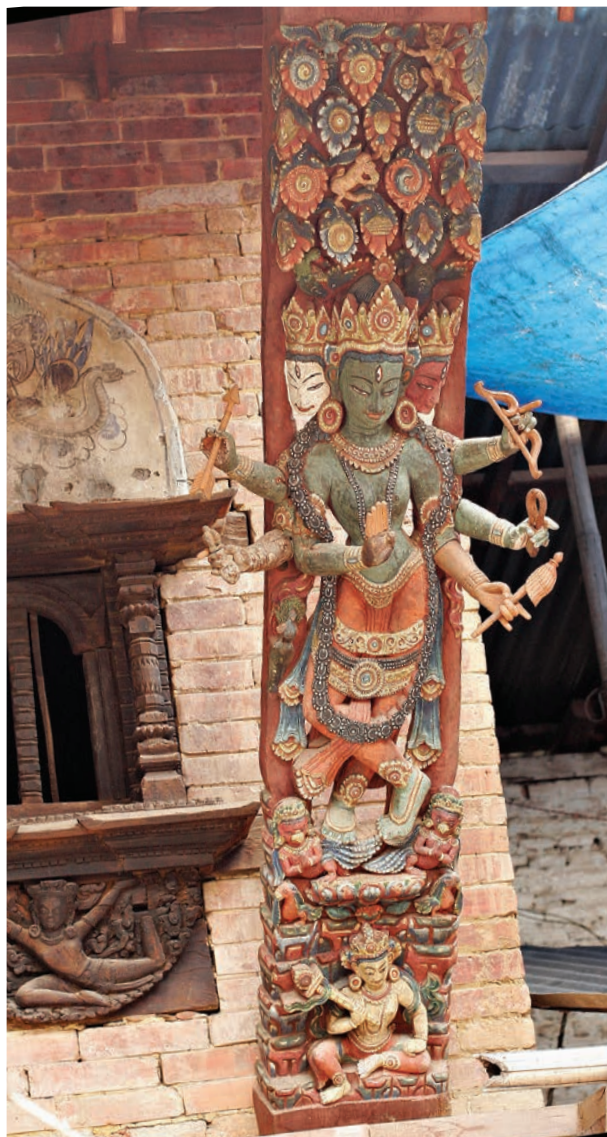
Existing struts of Itumbāhāh North Wing courtyard facade after cleaning. Photograph Rohit K. Ranjitkar, July 16, 2005
