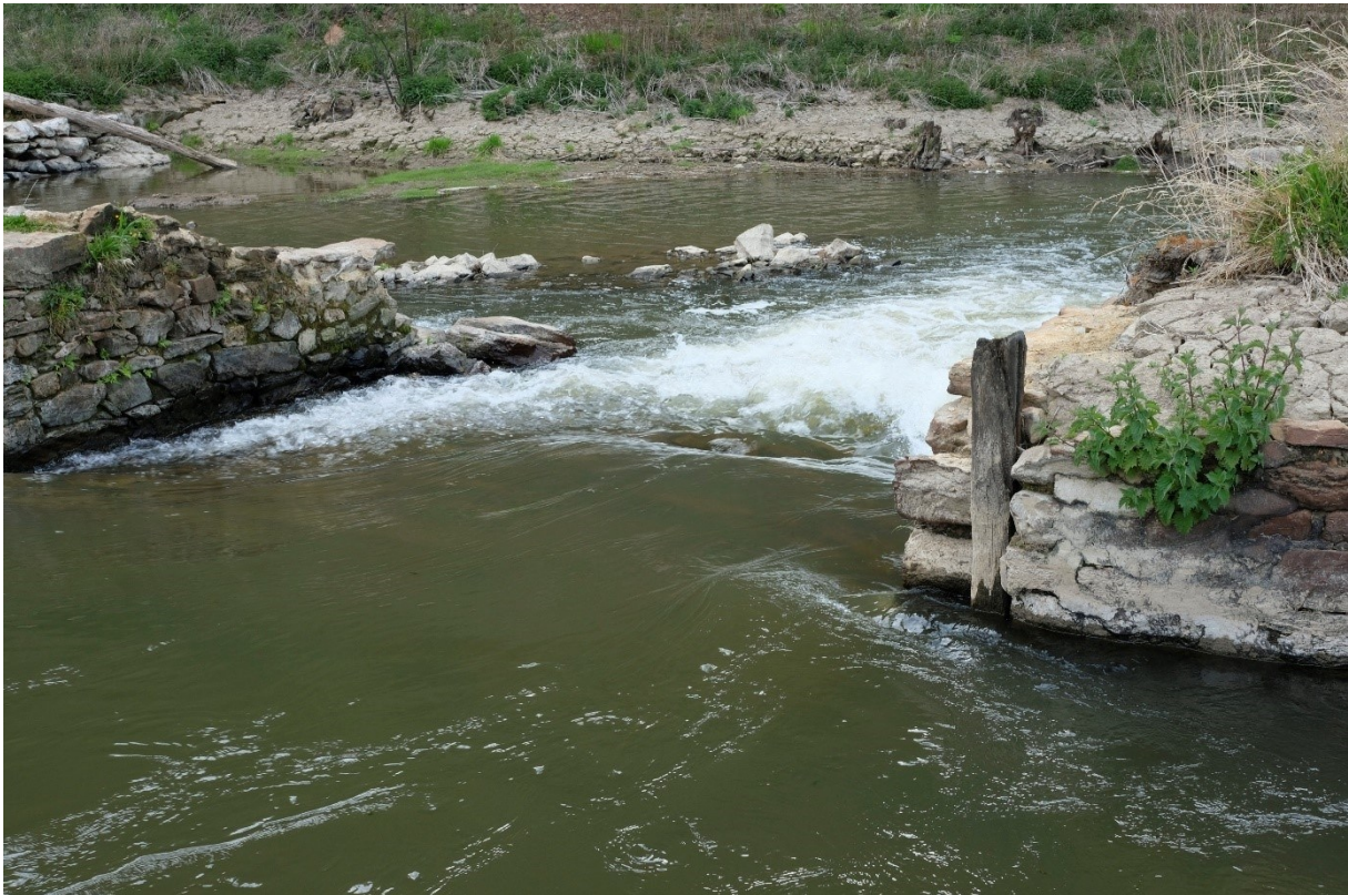
Figure 3 Alt Text: Photograph of an old small mill dam on the Sélune, which is broken in the middle, creating a rapid for kayakers
