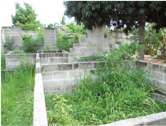
Housing under construction in Mapinga, a suburb of greater Dar es Salaam, Tanzania, 2019 © Schlimmer
