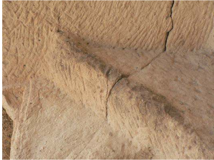
Fig. 4 Bench's irregularity to the northwest part of the nave with sledgehammer impacts (A. Lamesa).
