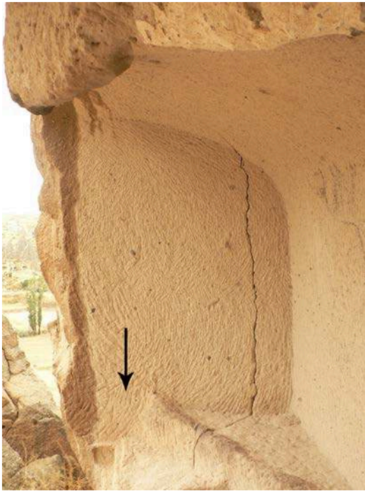
Fig. 11 Long-handled picks' impacts, west wall of the nave (A. Lamesa).
