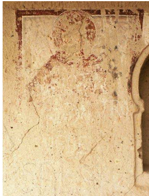
Fig. 9 The nave's painting destroyed by a niche (A. Lamesa).
