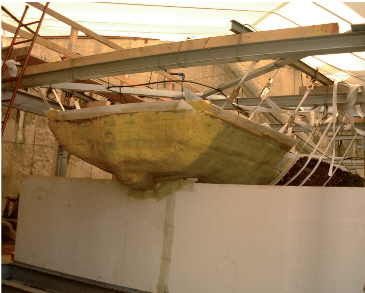
Figure 3. The fiberglass shell under construction on the prow of Napoli C shipwreck. Photo: G. Boetto, CNRS/CCJ.
