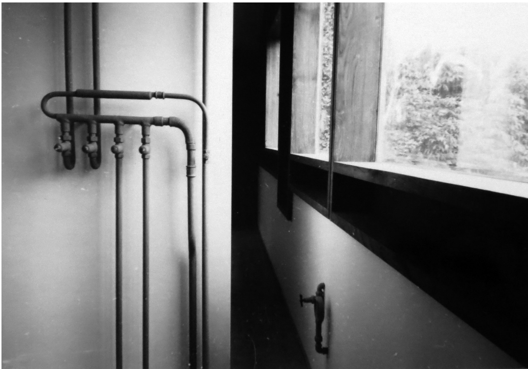
Figure 17. Heating system ducts
