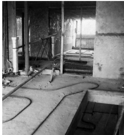
Figure 25. Apartment's coil (FLC L3-1-22)
