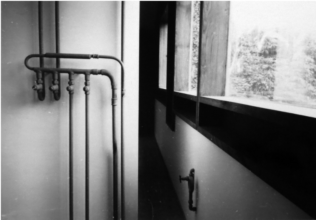
Figure 17. Heating system ducts
