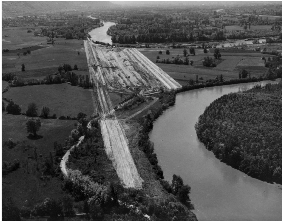
Fig. 5. The construction of a channel to cut a loop of the Isère River known as the “Bois Français” in 1968.
