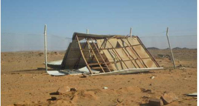
Fig. 29 : Debris of prefabricated housing unit
