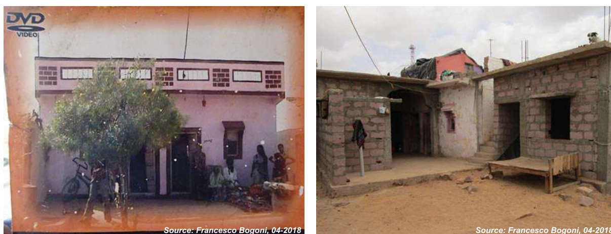
Image 25. 'One of the better' houses in Ramdevnagar before the project (left), and the worsening of condition as it was upgraded in the pilot project (right).
