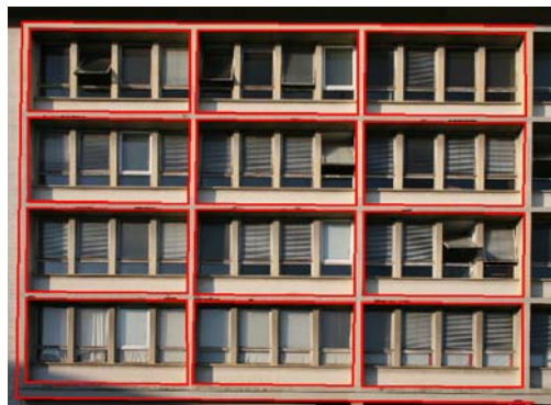
Figure 8. Part of the facade corresponding to the detected plane in Fig.7 (contours digitized in red)
