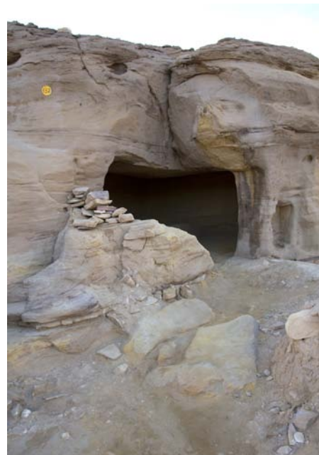
Fig. 29. Blocks from the collapse of the roof of IGN 132a
