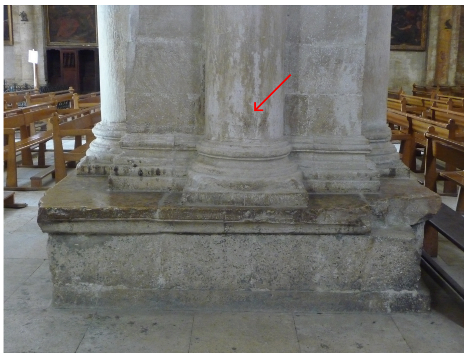
Figure 2. Photograph of the pier showing the location of the inscription by the red arrow (A. Hartmann-Virnich)
