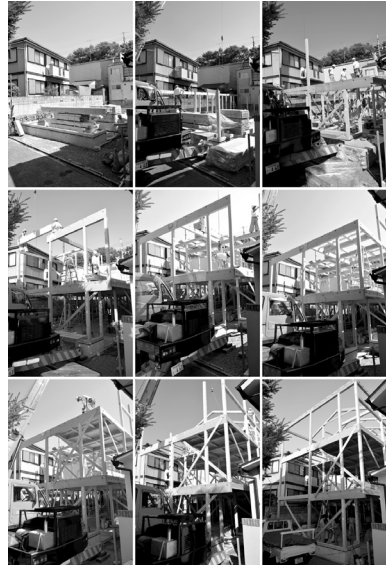
Fig. 17: Mikan, EFEO Centre Kyoto, the wooden structure mantled in 2 days, September 2013. Photographs ©Benoît Jacquet.
