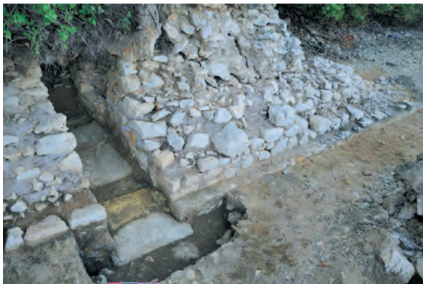
Fig. 8: Drainage canal built through the terrace wall (photo Ph. Groscaux, AMU, CNRS, CC)
