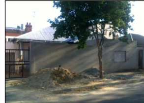
Blank wall: another example of a residential property being prepared for the installation of a spaza shop
