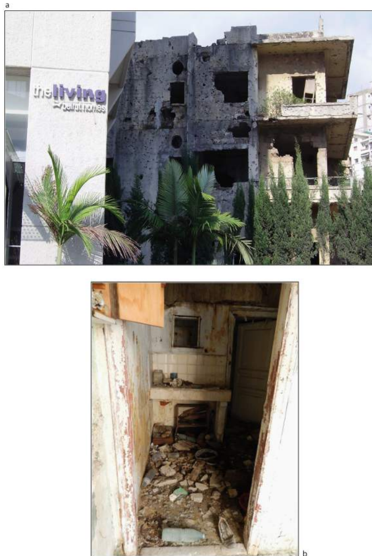
Figure 3: Beirut. Family homes destroyed by fire on the ancient Green Line of Damascus Street.
