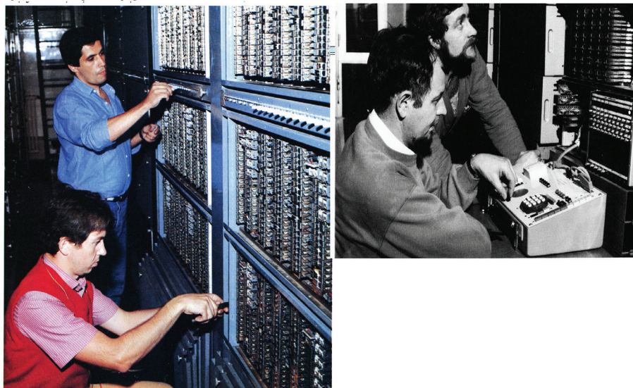
Figure 2. Technicians updating switching equipment. Source: Direction Générale des Télécommunications, “La France à 8 chiffres,” Revue Messages , October 1985, accessed July 1, 2023, https://drive.google.com/open?id=1P8sdhz6wpqL ENxiVZqDfiZg7JuyT-16l .
